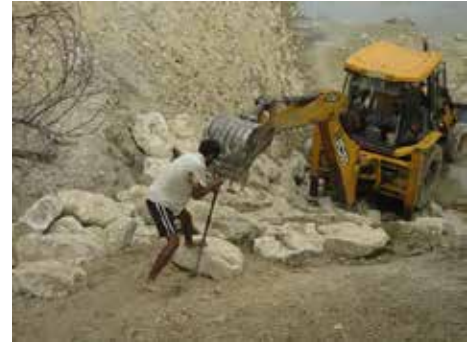
An even bigger challenge was a thick layer of very fluid sticky mud on the bottom of the old pond which took a lot of time to remove.
